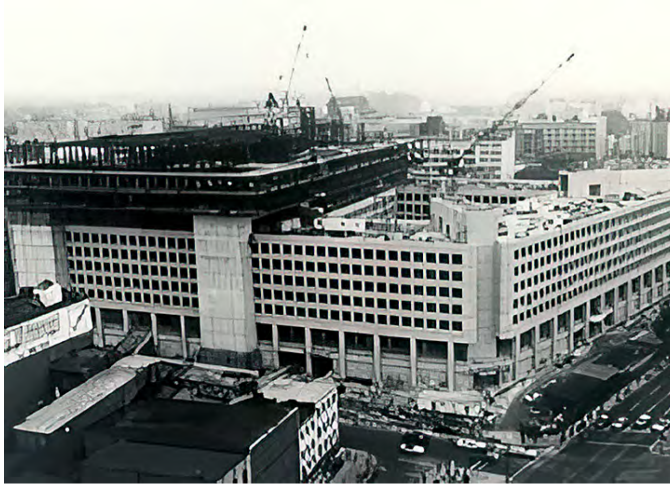
Under Construction, J. Edgar Hoover Federal Bureau of Investigation (FBI) Headquarters Ca. 1969 Federal Bureau of Investigation
